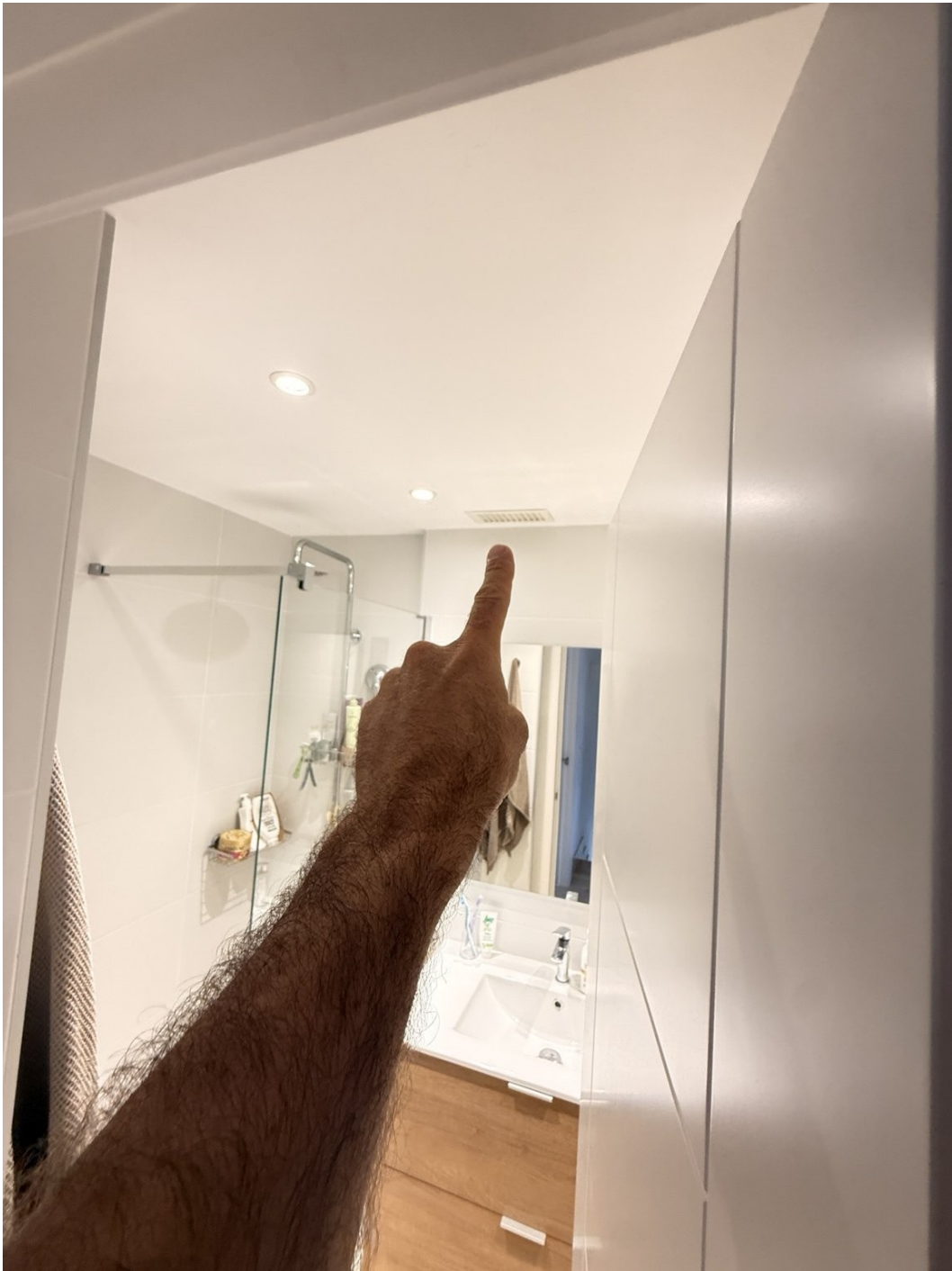
OBS-02 - Bathroom without adequate mechanical ventilation
