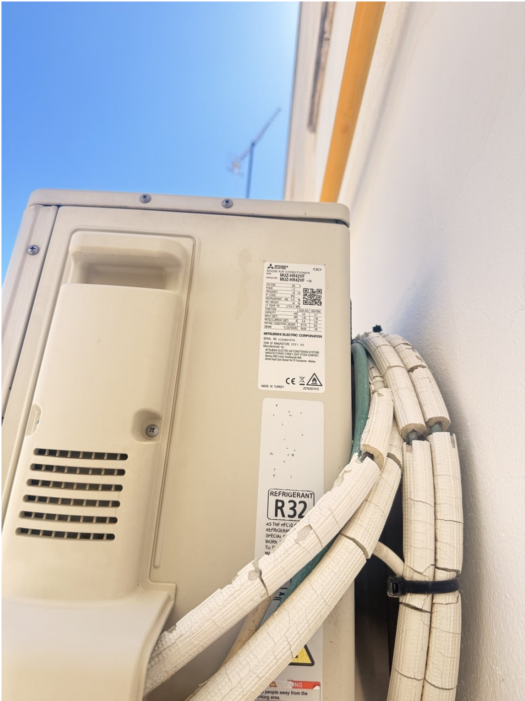
OBS-06 - Air-conditioning pipe insulation degraded
