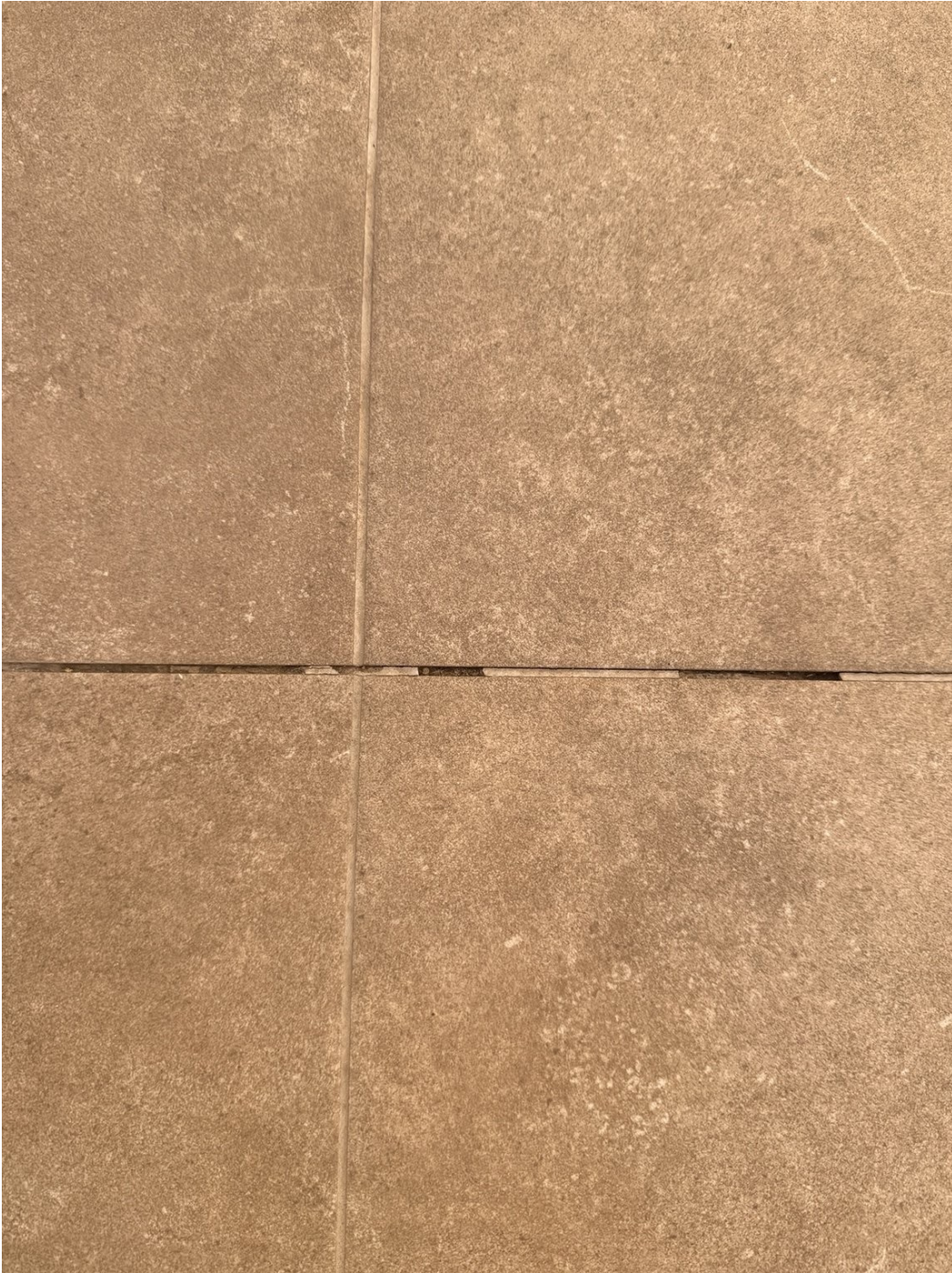
OBS-04 - Terrace tile grout joints to review
