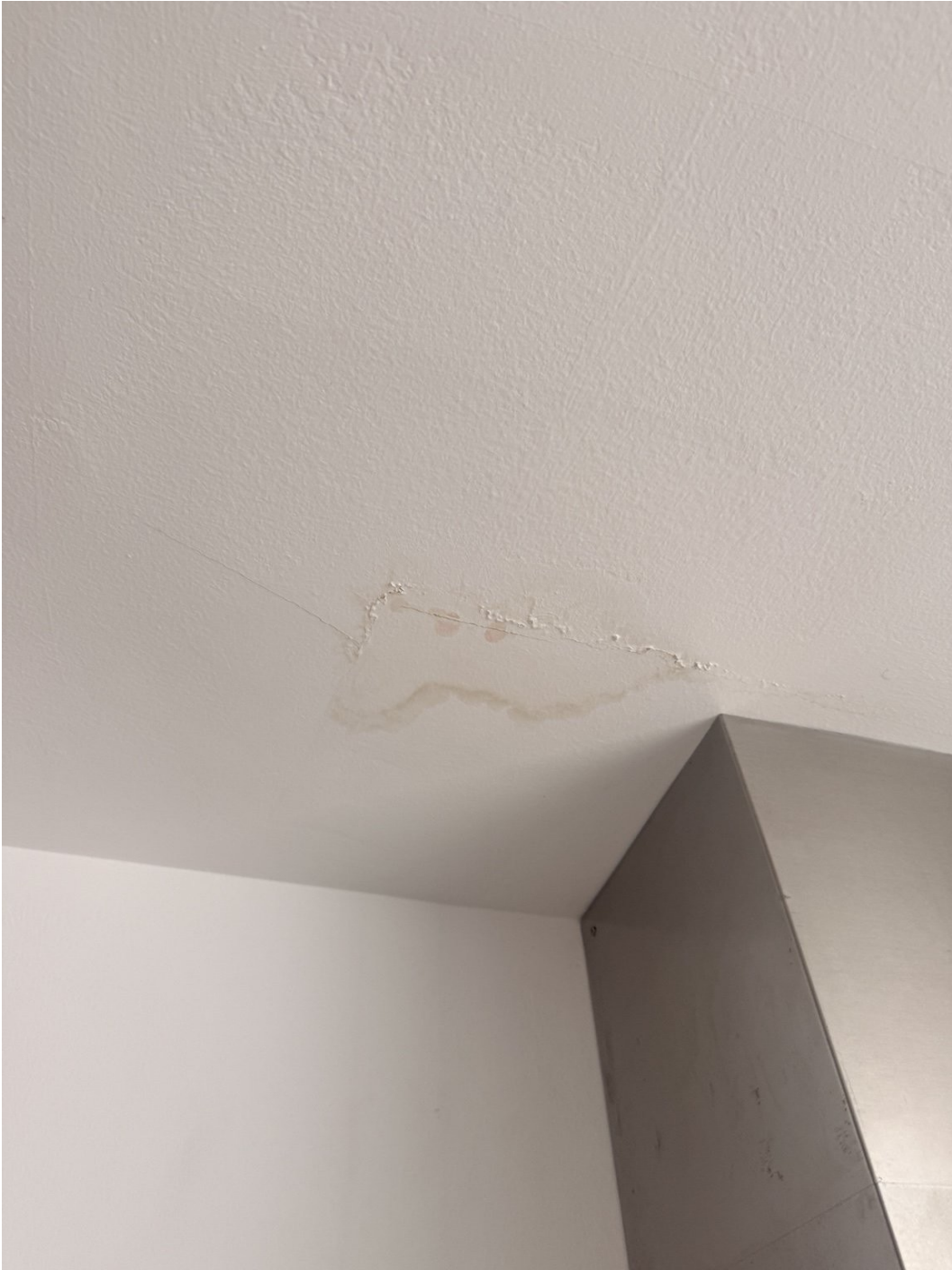
OBS-05 - Dry moisture mark at kitchen ceiling
