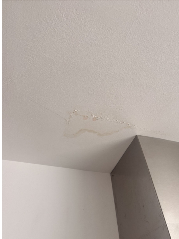
OBS-05 - Dry moisture mark at kitchen ceiling
