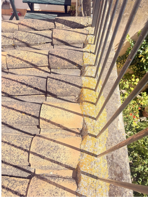
OBS-03 - Roof edge / flashing mortar requiring prompt repair
