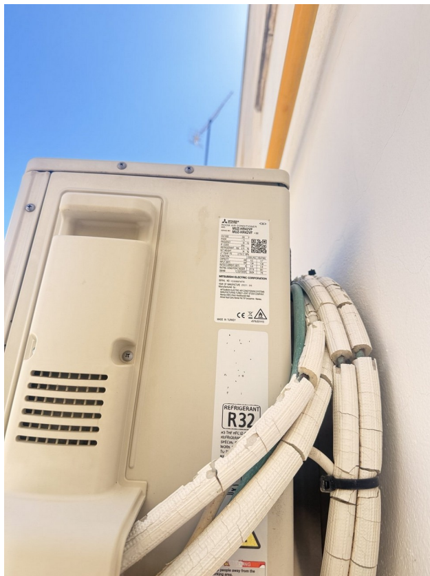
OBS-06 - Upper floor not served by air-conditioning
