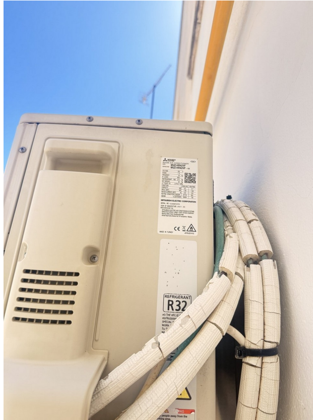
OBS-07 - Air-conditioning pipe insulation degraded
