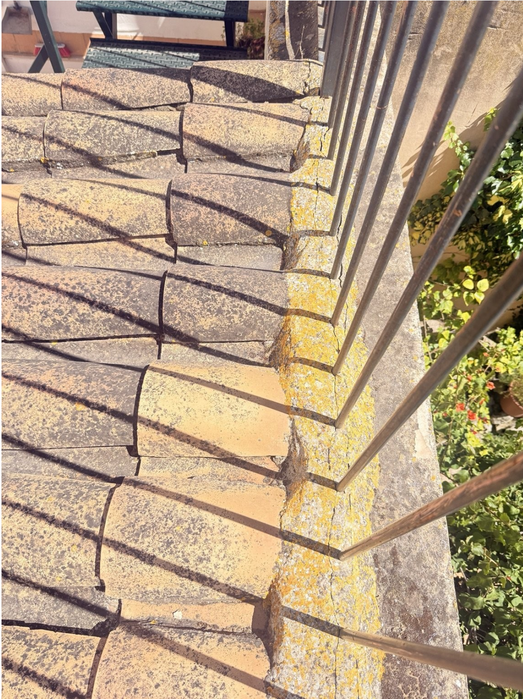
OBS-03 - Roof flashing / roof edge mortar requiring repair
