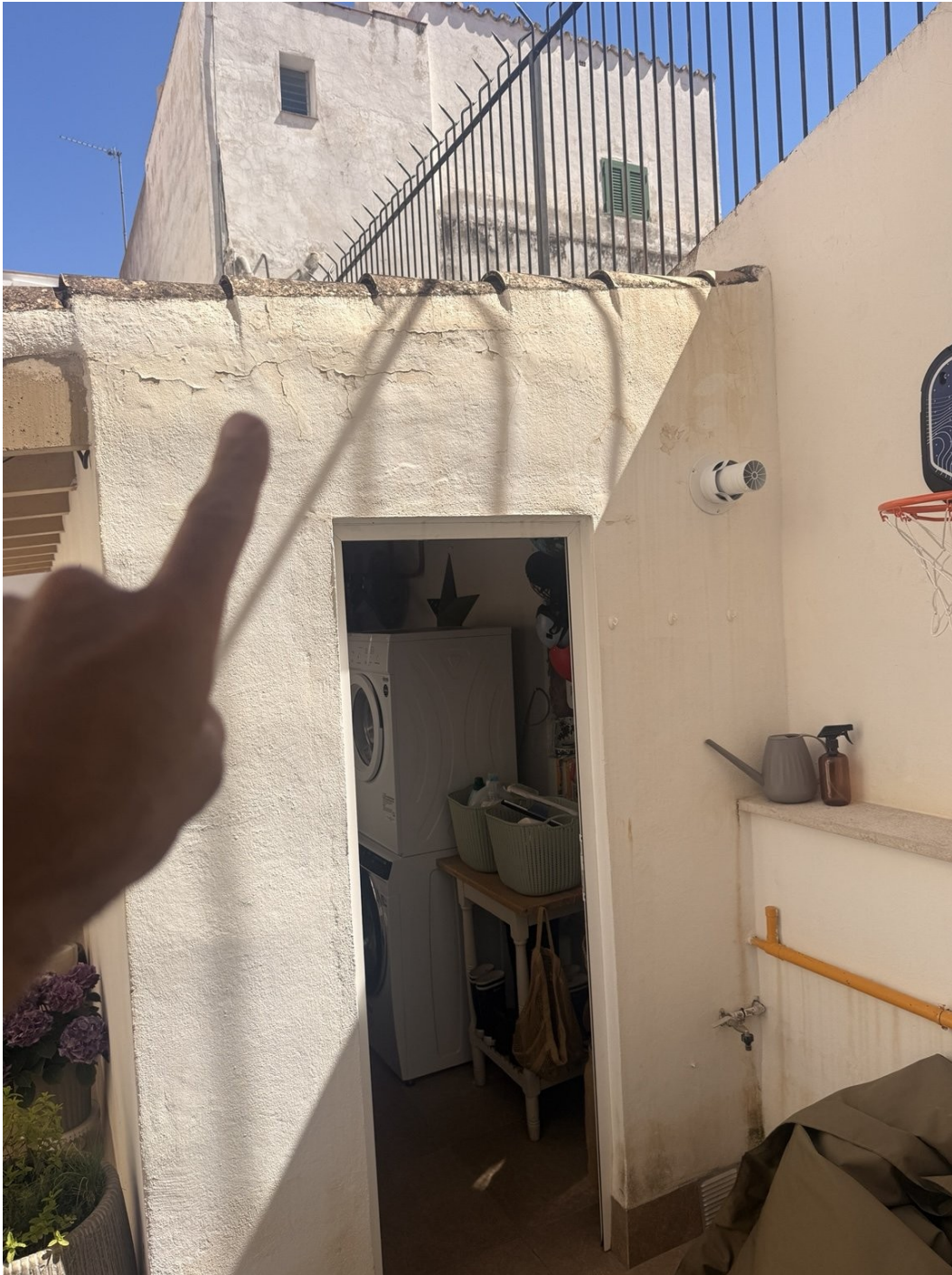
OBS-01 - Exterior utility room render cracking
