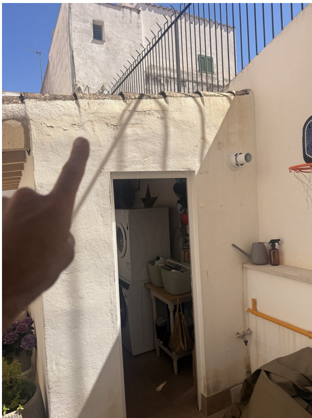
OBS-01 - Exterior utility room render cracking and surface deterioration
