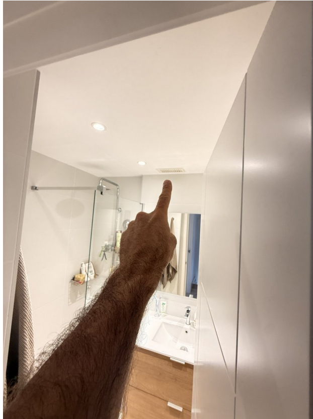
OBS-02 - Bathroom without adequate mechanical ventilation
