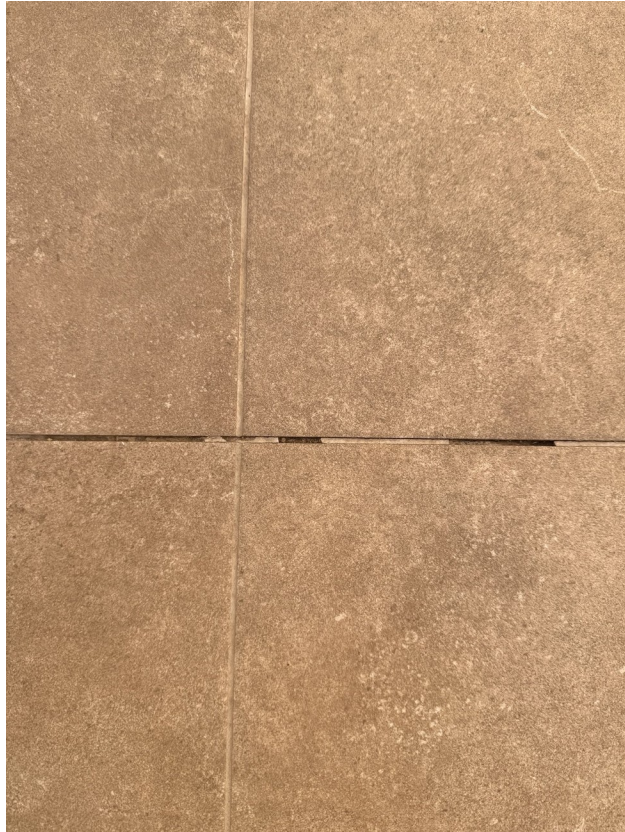
OBS-04 - Terrace tile grout joints to review
